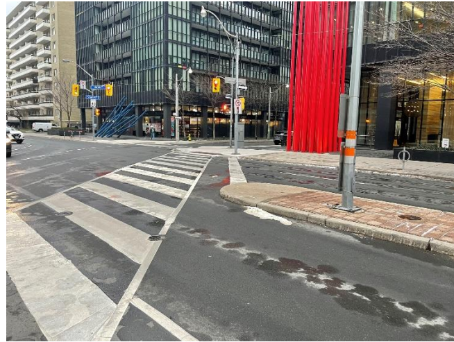
Channelized island at the Northeast corner of the intersection looking southwest toward Charles Street East showing the angled crosswalk on the north leg of the intersection.
